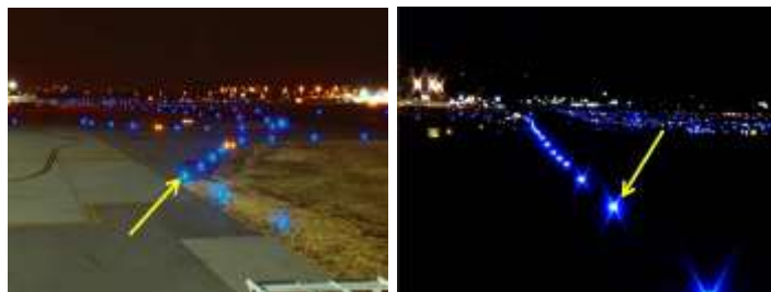
Gambar 6. Taxiway Edge Light
